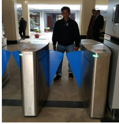
Access control system
